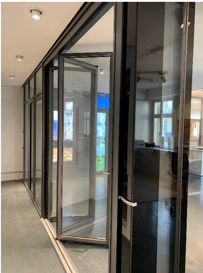
Figure 2: A Solarlux folding system was integrated directly into the Hueck facade (source: Hueck)
